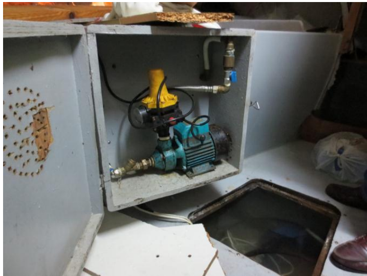
Figure 5.4–Damages on bilge pump
