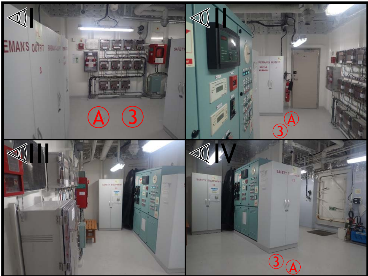
Figura 6. Interior del local Fire control room .
