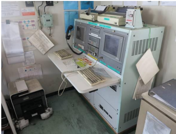
Figure 2.2 – Bridge Communication equipment
