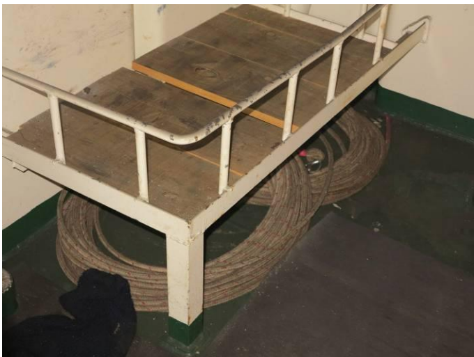
Figure 8.12 – Type of fire line guides not used
