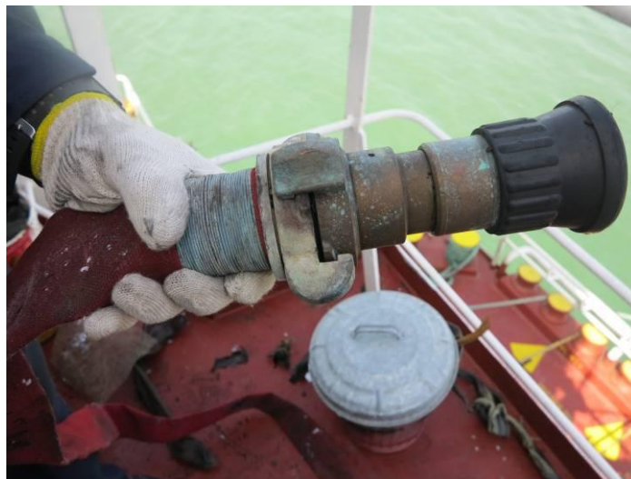
Figure 8.10 – Type of fire nozzle used
