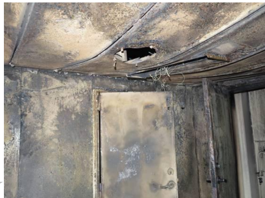
Figure 8.3 – Cabin ceiling buckled due to heat
