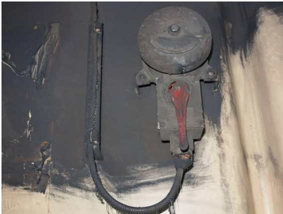
Figure 8.6 – Melting of plastic on fire alarm
