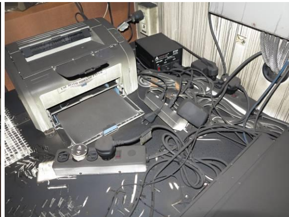
Figure 8.9 – Captain Office Smoke deposits
