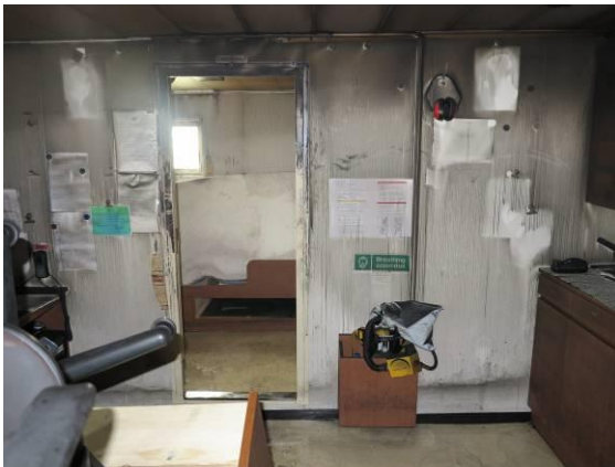
Figure 8.8 – Captain Office Smoke deposits
