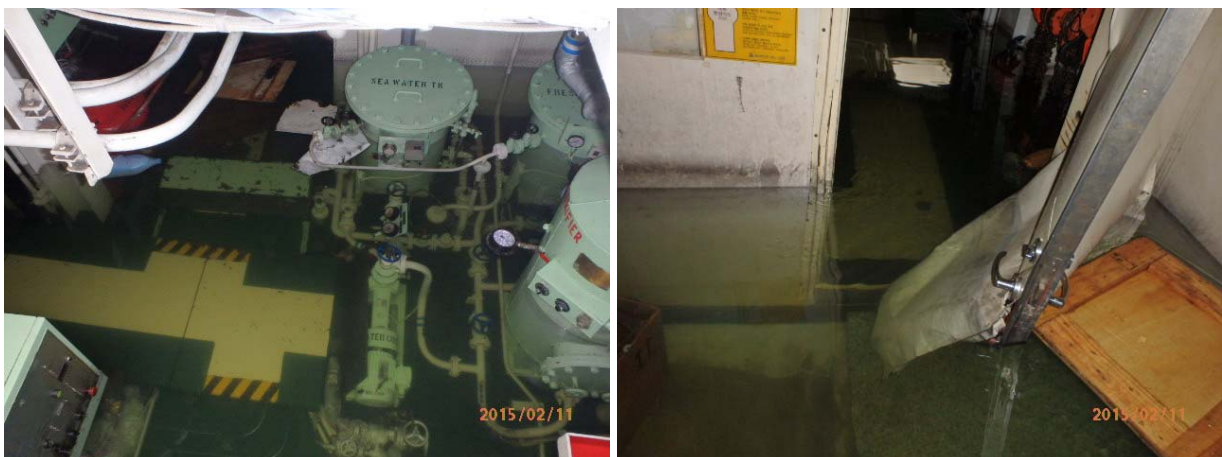
Figure 6. Flooding in the engine room.
