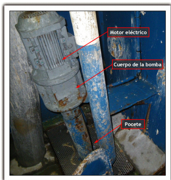
Figure 4. Stern sump pump located on the starboard side of the fishing area
