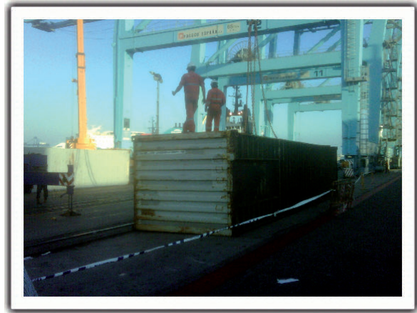
Figure 11. Container removal work carried out by the company in charge of the salvage operations on 12 June
